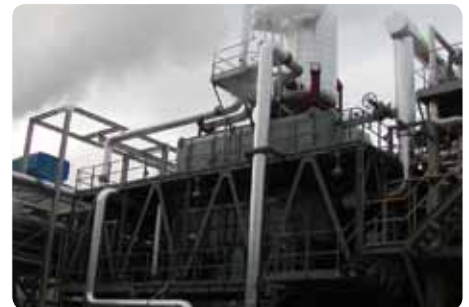
· 10 ton/h Absorption Heat Pump Installation [Korea]
